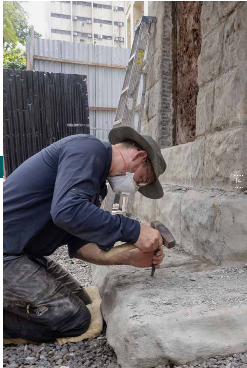
Right: Technical manager for our work department, Peter Dickerson, preparing the Freetown memorial as construction begins, photo Lansana Mansaray.
