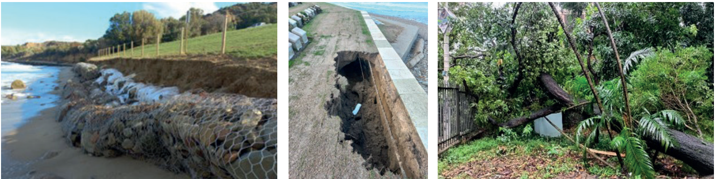
Storm damage: soil collapse at Anzac Commemorative Site (Türkiye) (left) & Ari Burnu Cemetery (Türkiye) (centre) due to sea erosion; tree fall adjacent to Chittagong War Cemetery (Bangladesh)
