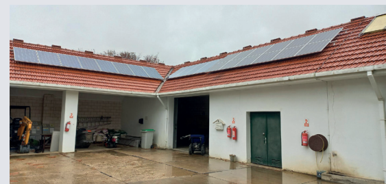
Anzac Base Site (Türkiye) (installation needs repair after damage by wildfire)
